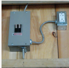
Panel Box & Receptacle
